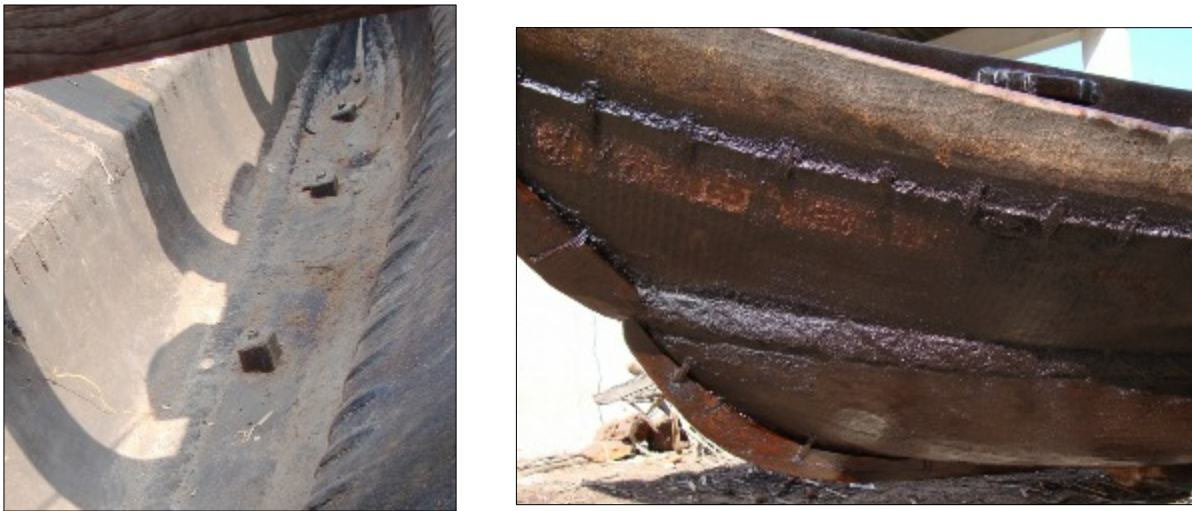
Figure 4. a) barely visible stitches inboard between the underbody and garboard. Bolts fasten a false-keel along the centreline of the underbody. Fish Road; b) well-maintained two-strake pirogue with false-keel attached by stitches. Cova. Author.
