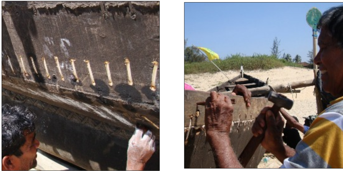
Figure 12. Outboard: a) grooves span a new split and an old seam. The surface is made good below with hand-applied chunam ; b) ends of wedges are trimmed and battered. Fish Road. Author.
