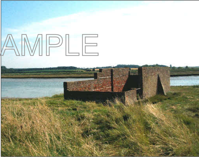
The now roofless brick warehouse. Before World War II it was still used by Winch's barges, including the Bluebell, to store: hay and straw awaiting shipment; and offloaded coal.
