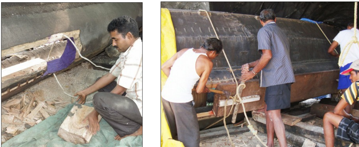
Figure 14 Repair to the underbody of a pirogue involves offering up new work numerous times: a) Siridau; b) Benaulim. Author.
